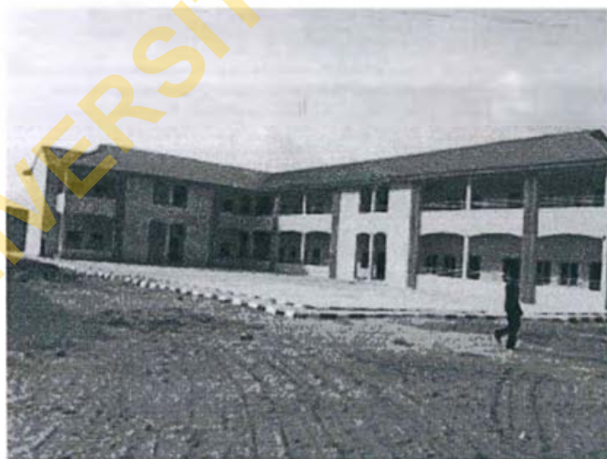
Figure 4: Construction of Model School Building, Igbokoda, Ilaje LGA Source: Ondo State Government, 2013
